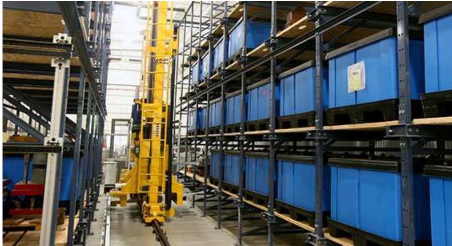
Image 5. Complete Automated Pallet Storage and Retrieval System
